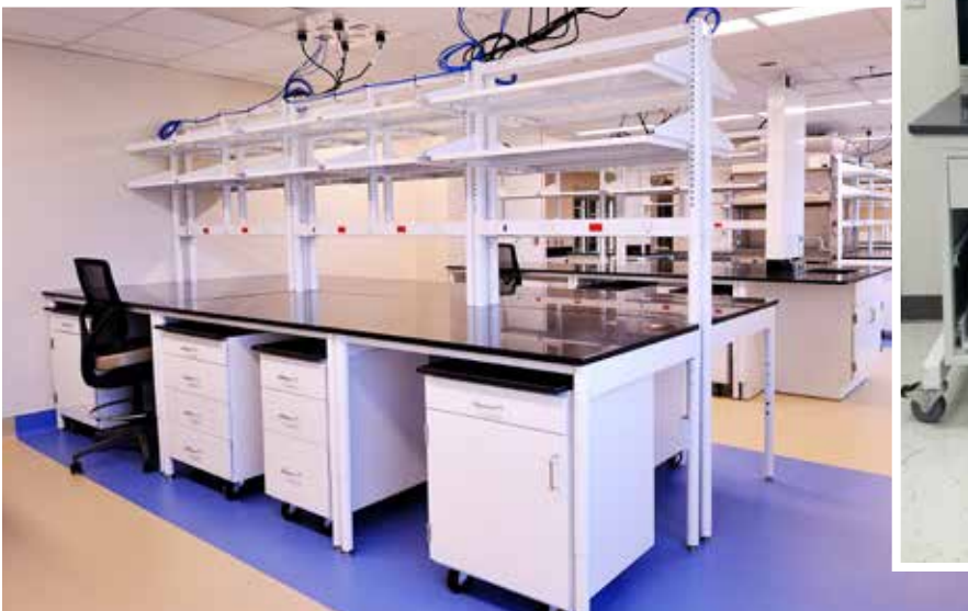
Enterprise pre-plumbed & wired movable benches
